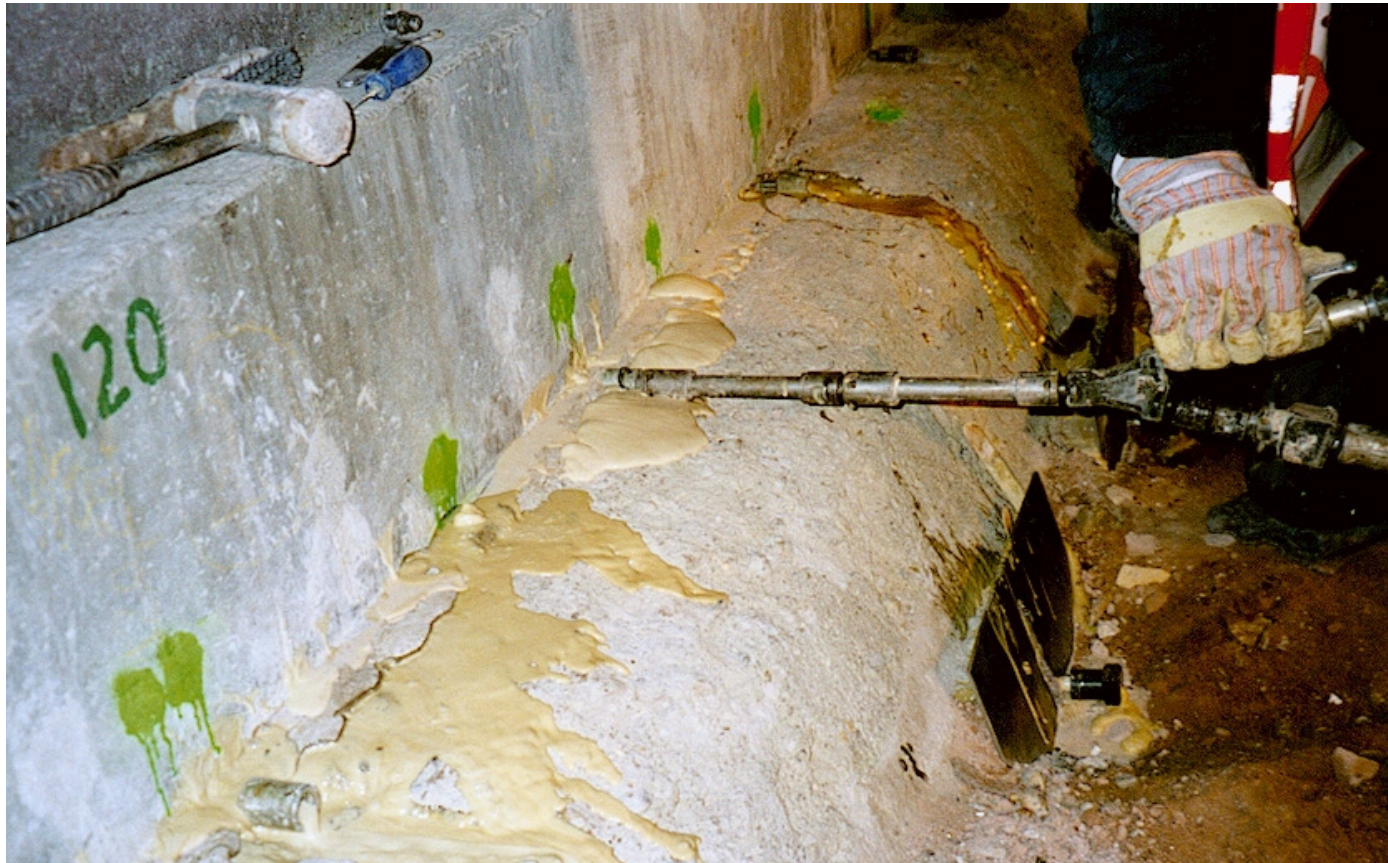
Injection between the layers of the slab structure at high speed line from Hannover to Berlin, Dallgow
