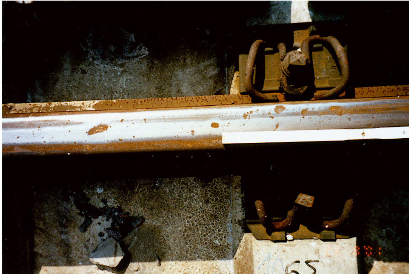
Rail head deterioration after grinding
