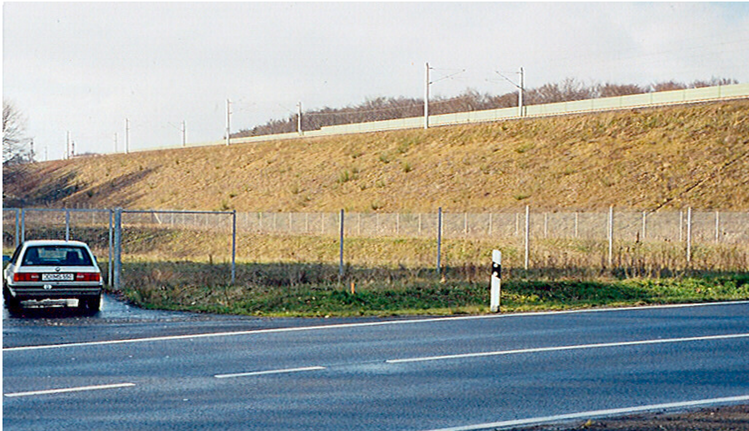
Dam with extreme settlement (high speed line from Colongne to Frankfurt/Main, km 72,602-72,692)
