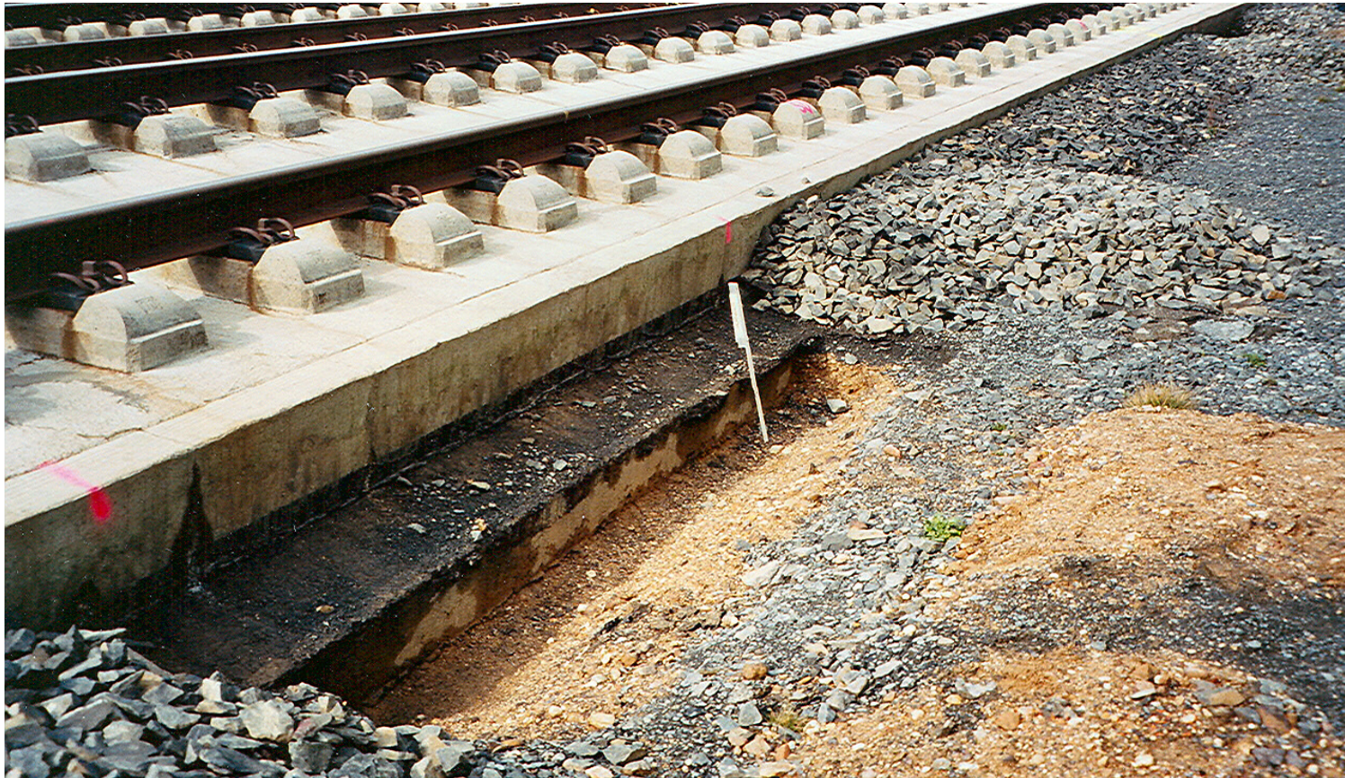
Slab track without visible defects (high speed line from Colongne to Frankfurt/Main, km 72,602-72,692)
